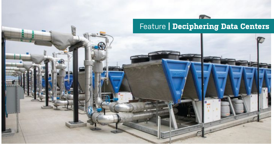
This is the chilling portion of a closed-loop colling system for a data center. The blue air conditioners cool a pipe containing water, which is then used to cool the air coming off the servers at the Sabey data center in Quincy, Washington. | RYAN HALL PHOTO
