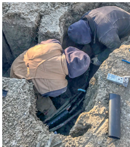
The hole has been cleared and the crew is beginning repairs to the cable.
