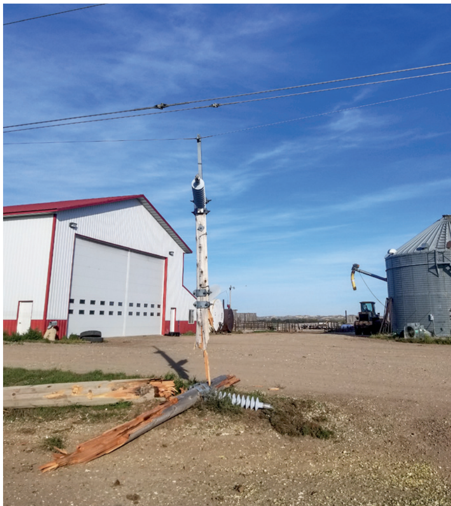
Basin Electric Power Cooperative's pole was badly damaged during a hit-and-run accident. Don't let appearances fool you – the line is still energized.
